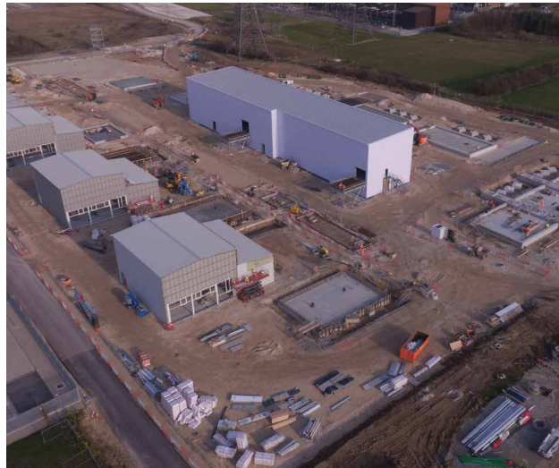
Aerial photograph of the onshore substation
