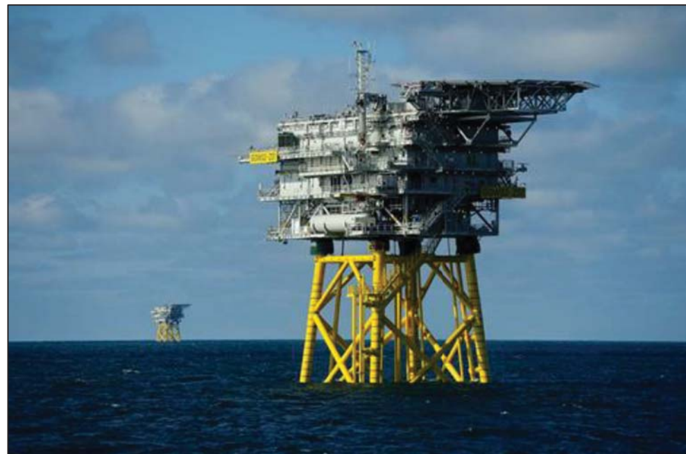
Figure 3.9 Offshore substations at Gode Wind offshore wind farm.
