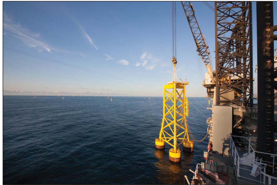
Figure 3.4 A jacket foundation with suction buckets being installed at the Borkum Riffgrund One offshore wind farm.
