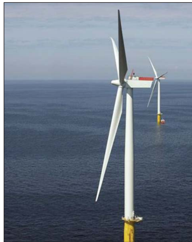
Figure 3.2 Wind turbines at Walney offshore wind farm.
