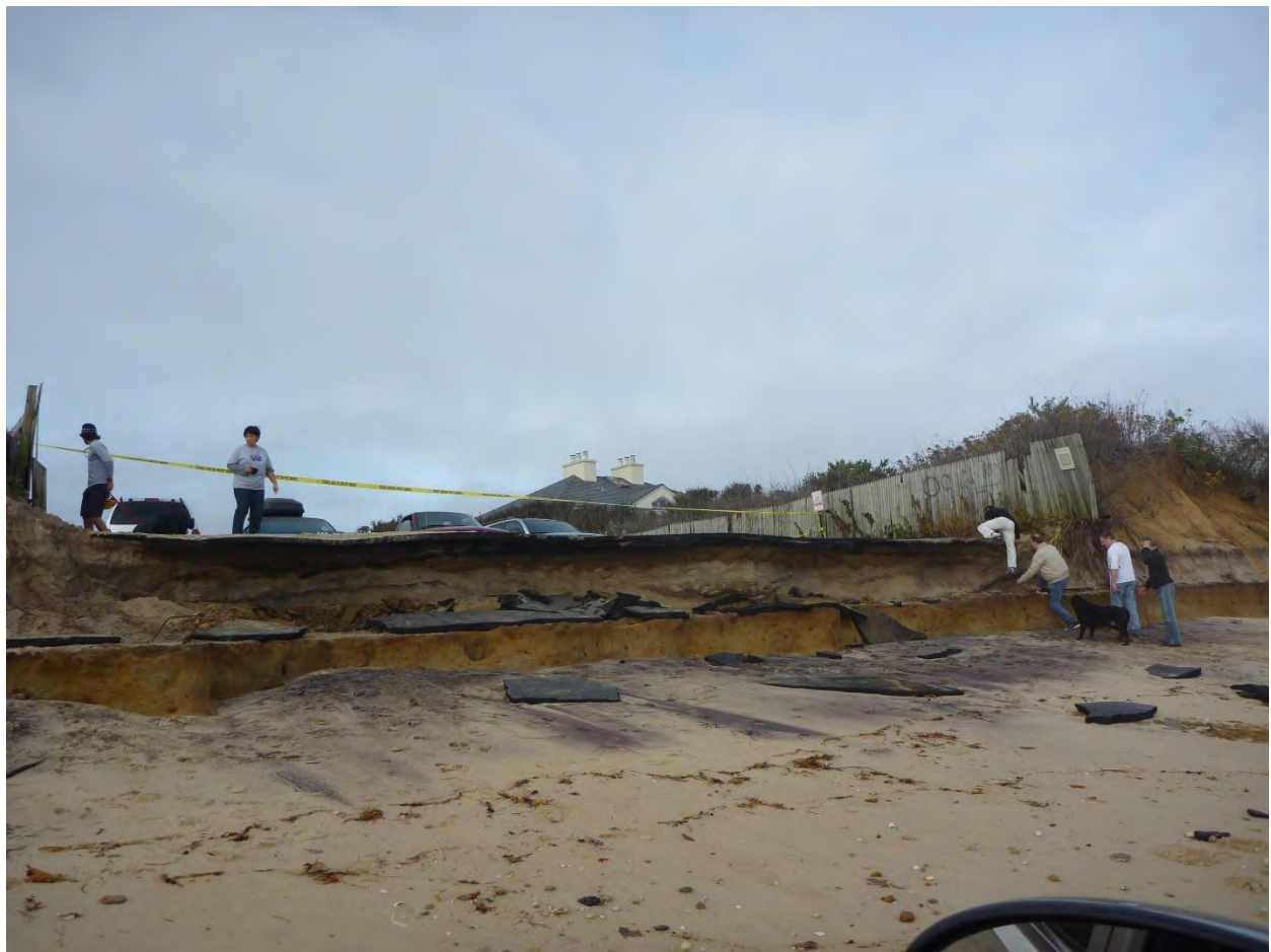
Figure 5: Post storm photographs taken on 2009-11-12 reveal the headland soils at the seaward end of Beach Lane in Wainscott.
