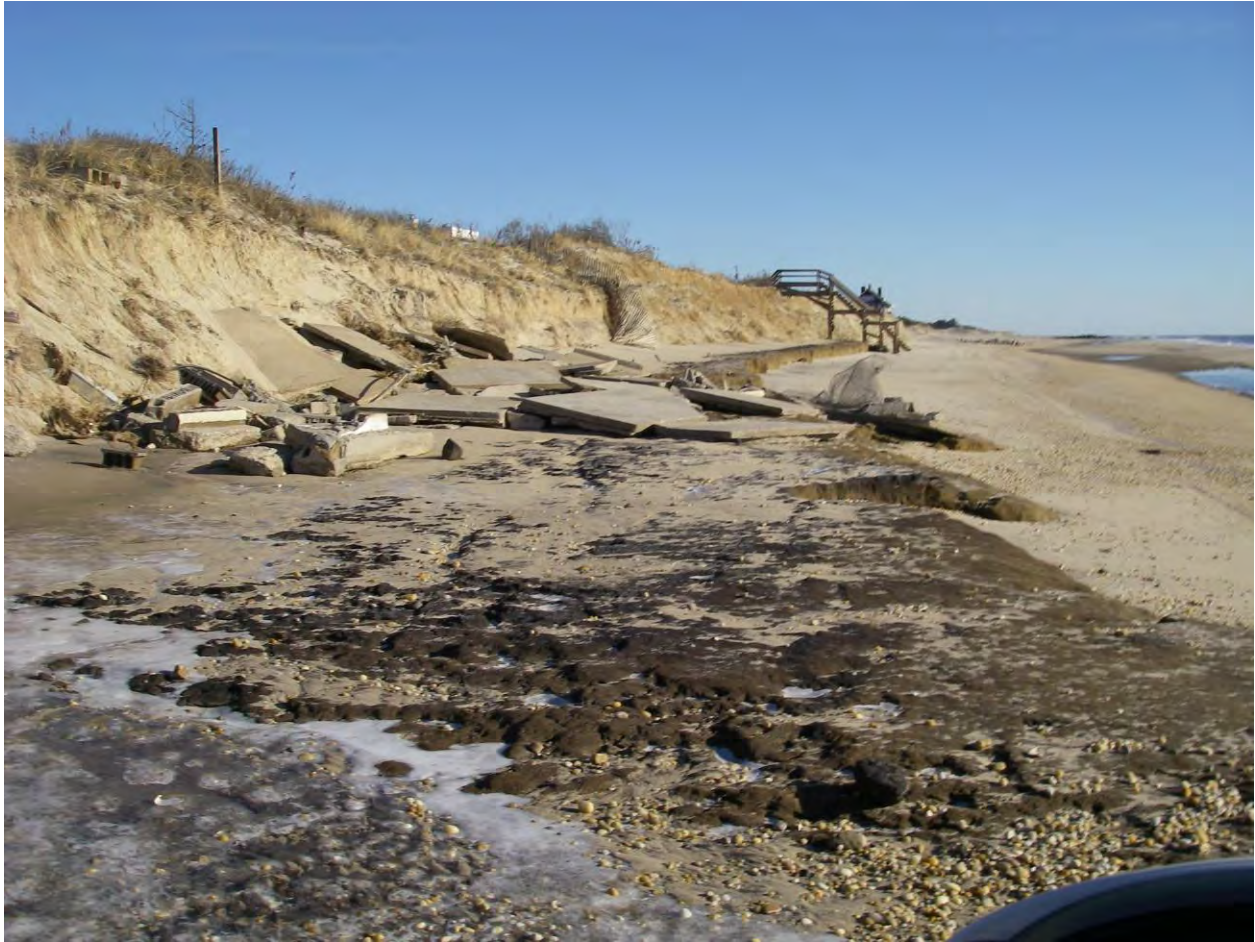
Figure 6: An immediate post storm photograph of the beach east of the Beach Lane area taken after a coastal storm on 2008-12-22. The unconsolidated sand has been eroded off the top of the more resistant headland soils. Horizontal distance is over twenty feet in the foreground.
