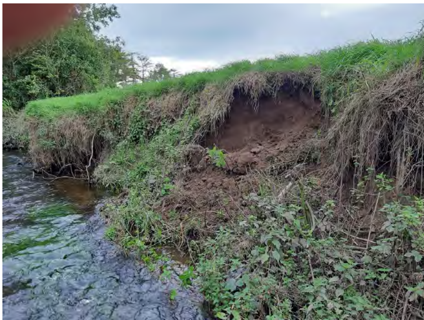
Photo 7: Clyda River. Bank Erosion
