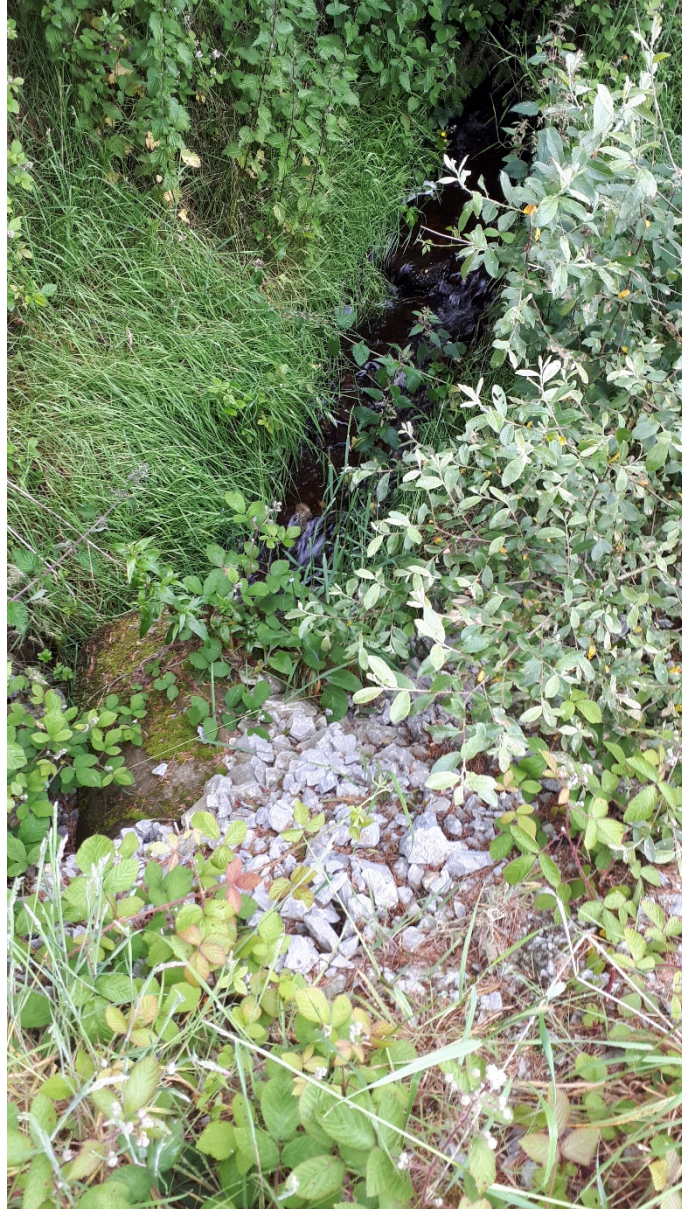
Viewpoint looking upstream of the location of the proposed culvert reconstruction over the Toor River
