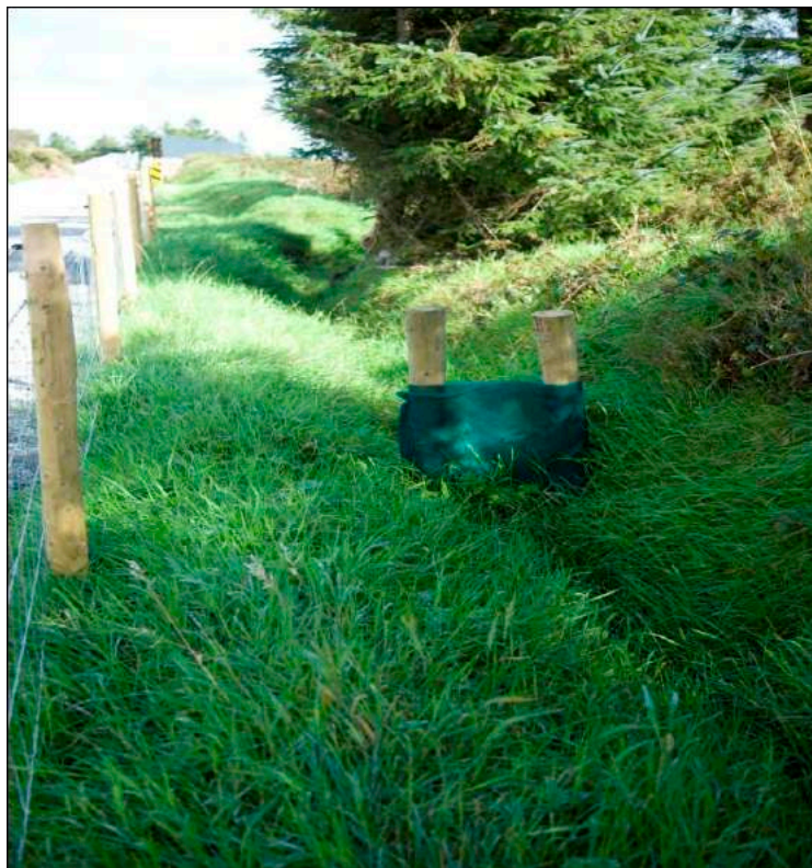
Figure 4: Silt Trap across Grassed Swale
