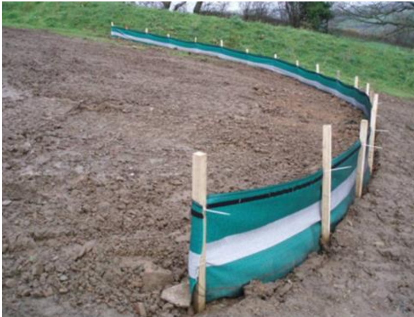
Plate 5.4: Typical Silt Fencing
