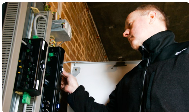
Small boxes like this one is what will create the intelligent power network. They were first installed in 2007 and by the end of 2009 more than 400 transformer stations will have been automated.
