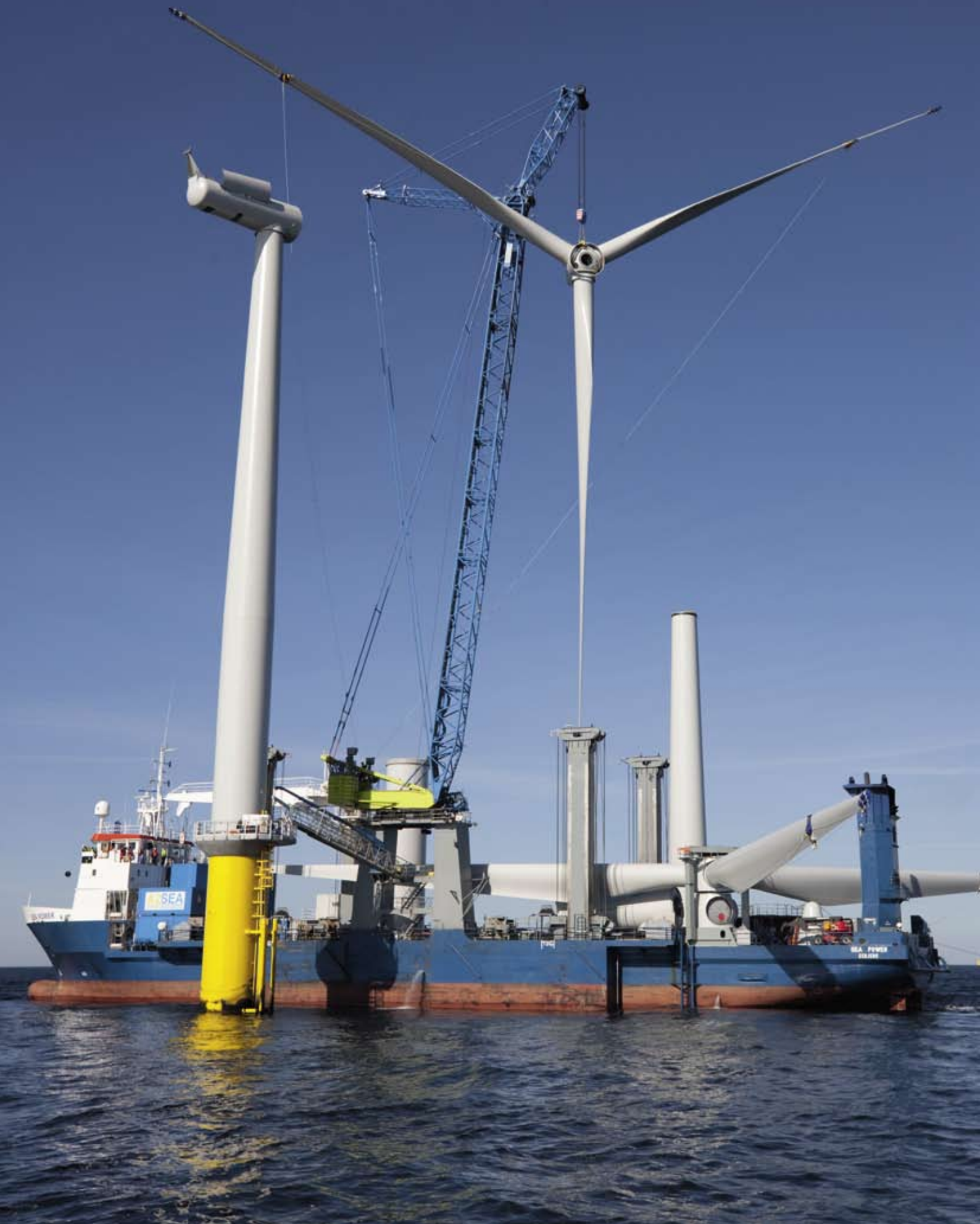
Installation of foundations and wind turbines at Horns Rev 2 offshore wind farm, which is located 30 km off Blåvands Huk.
